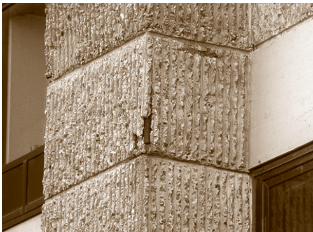
Reinforcement corrosion and spalls in béton brut (“raw” concrete), an aesthetic feature commonly used by architects of the Brutalist tradition, among them Paul Rudolph. His Art + Architecture Building at Yale University recently underwent a major renovation.
