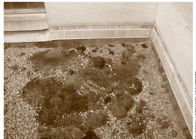
Organic growth and debris on the built-up roof of a Modernist structure. The materials and techniques of Modern architecture allowed for rapid and prolific construction, which resulted in a historically unprecedented volume of new structures during this period.
