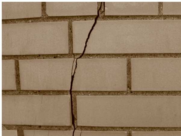
Vertical crack in a glazed brick façade. A major characteristic of Modern buildings was the shift from façades with thick, massive walls and proportionally few windows to slimmer wall construction and more widespread use of glass.
