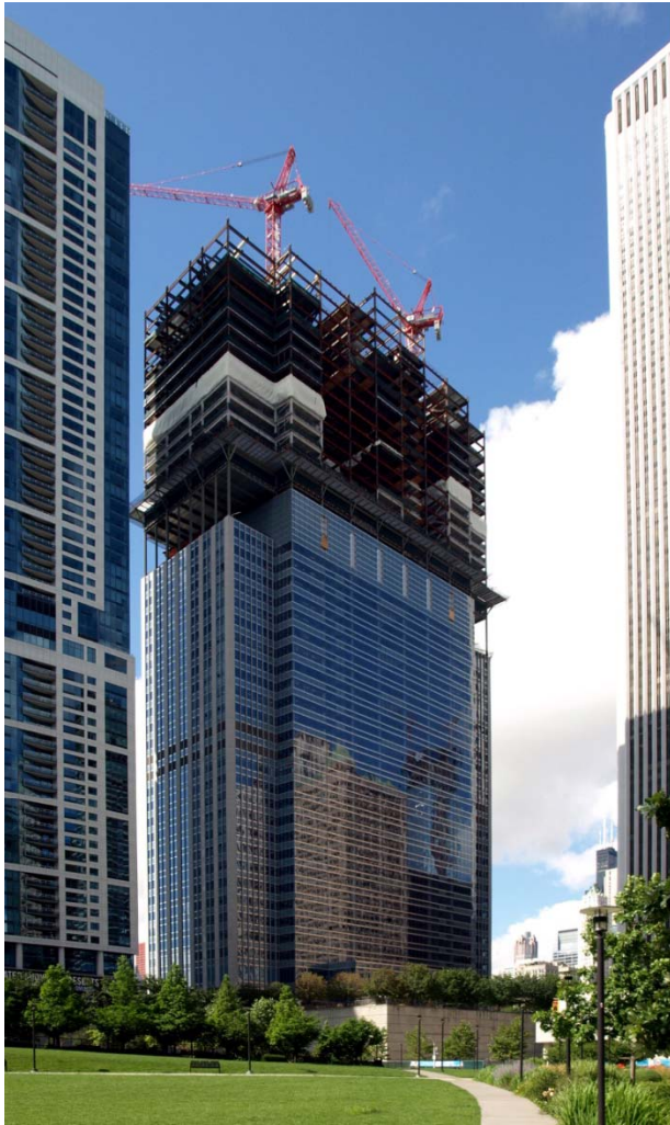
A construction photo from August 2008 shows the vertical expansion rising above the initial building—all while the building and company
